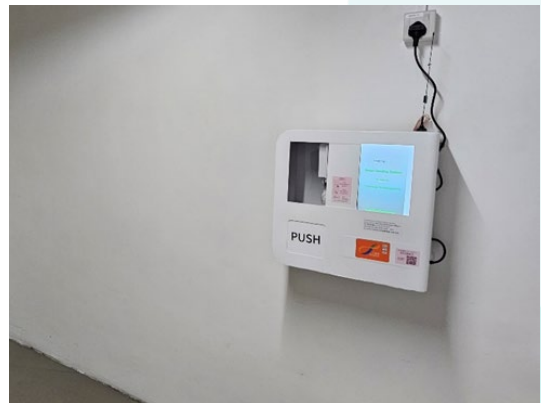
Pad vending machine installed outside YIA G/F female restroom.
